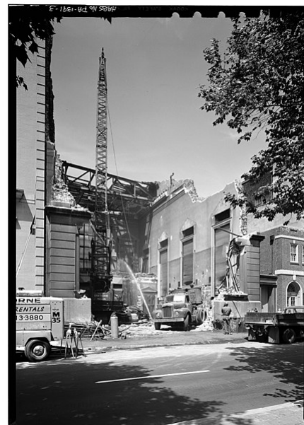
Demolishing the Bank of North America's building at 305–307 Chestnut Street, Philadelphia (1959 or later)
