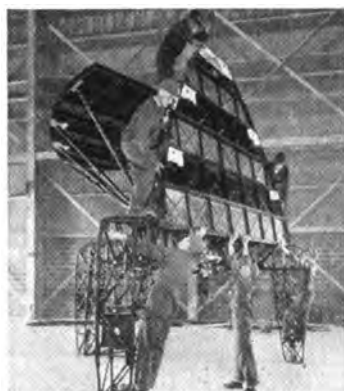
Here, the crew has assembled the antenna tripod. With a block and tackle attached to the radome crown piece, they are positioning the antenna base.
