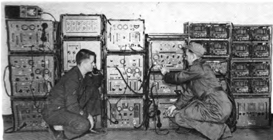
Assembled above is terminal equipment, telephone AN/TCC-7 and radio terminal set AN/TRC-35
