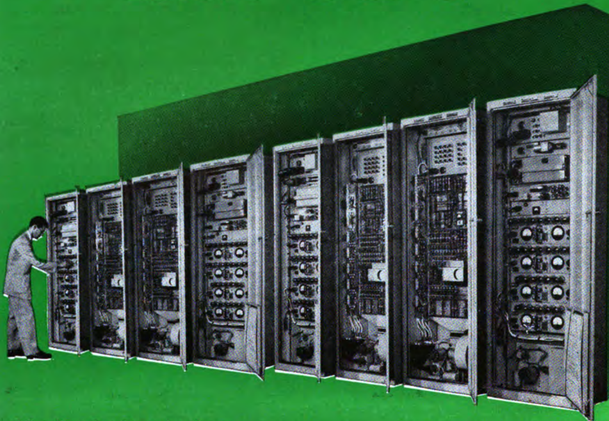
*Coordinate Data Transmitter System
