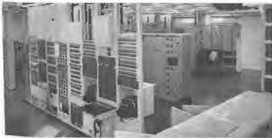
Pictured here is the Telegraph Test position of the Transatlantic Telephone Cable.
