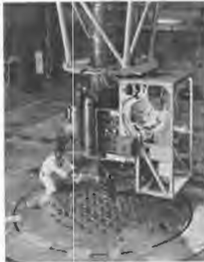
A huge, lead-shielded chamber for loading uranium fuel into the atomic energy reactor hovers over the "core" or heart of the reactor sunk deep beneath the ground. Heat from the atomic "furnace" is used by the experimental power station to generate electricity.
