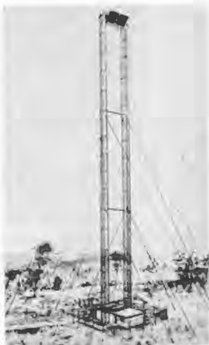
Pictured above is a drawing of Western Union's new self-supporting microwave tower with "fly swatter" reflectors. A reflector catches the beam and directs it to receiving equipment at the bottom where the signal is amplified and angled upward to another reflector which flashes it on to the next station. This is the tower now being installed on W.U.'s microwave beam system extension to Cincinnati and Chicago.
